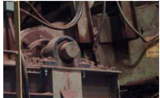
The brick company runs QM tapered adapter bearings in the clay re-claimer. Half the time was required to install them compared to the brand previously installed.
