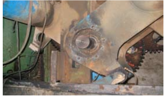
With a limited amount of shaft to work with, QM Bearings was able to come up with a solution for the mill that limited their downtime to less than one day - including the time it took to "torch off" the failed bearing.
