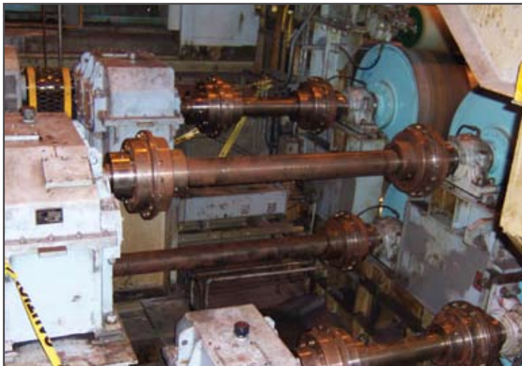
An evaluation of the elastomeric coupling was done on the plant's continuous descaling cold mill looper drive, a double-driven, high torque winch assembly.
