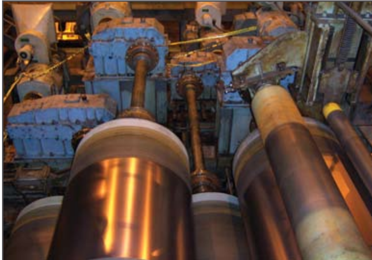
An elastomeric coupling replaced a gear coupling in this state-of-the-art coil processing facility.
